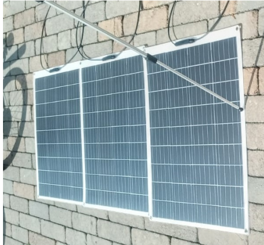
Figure B.3: Initial test of 3 PV commercial flat modules
