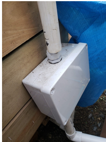
Fig. 10.23.: Power supply junction box.
