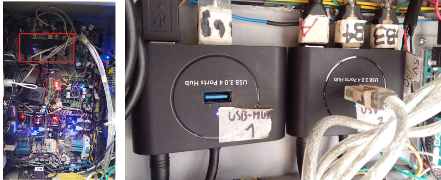
(a) Overview of the USB hubs' distribution on the electrical cabinet. (b) Detailed view of the four USB 3.0 port hubs.
