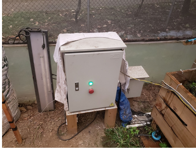
Fig. 10.18.: Electrical cabinets' location.
