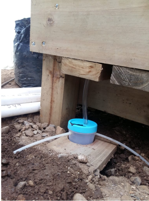
Fig. 10.13.: Assembly of the pH measurement system.
