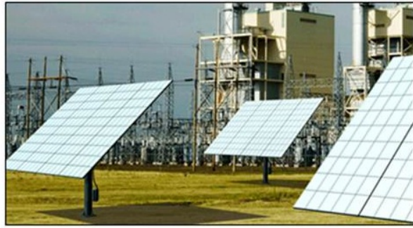
Figure 2.1: CPV module manufactured and power plant installed by SEMPRIUS. [27]
